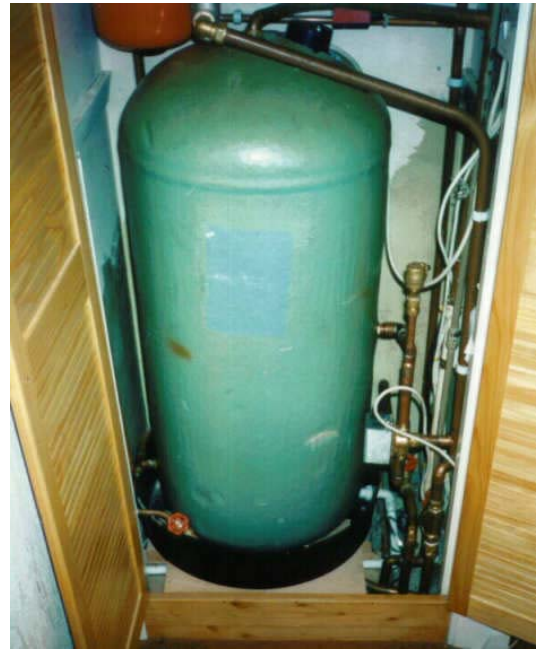
A fully plumbed in cylinder tank sitting in the cylinder tray (tray is black in this installation) with water vent pipe (white) flowing under tray from right to left and out through the wall
