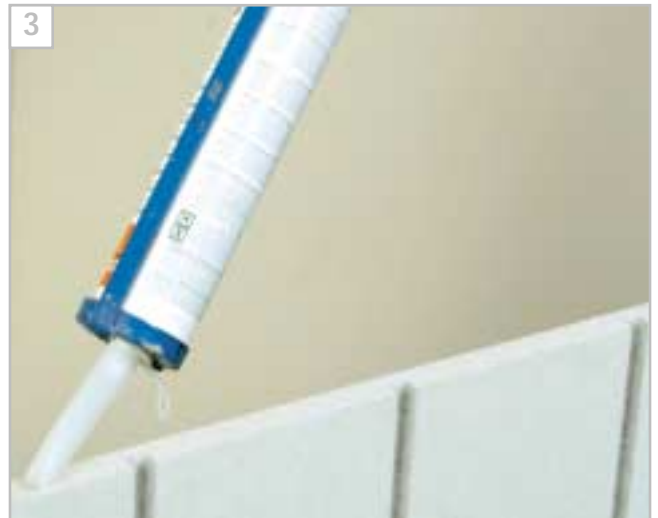
Apply a 3mm bead of adhesive to the end returns of the first panel
